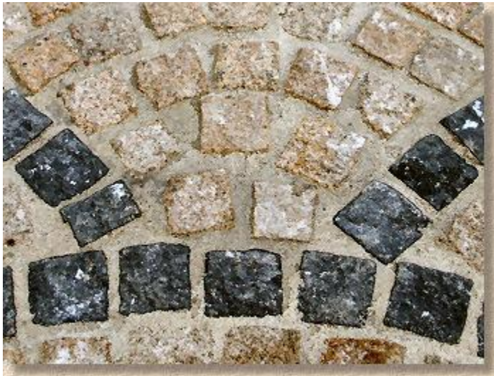
Lack of cutting or wedge-shapes results in wide joints
