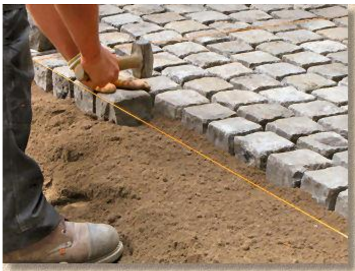
Setts are laid to a taut string line to guide accurate alignment and level
