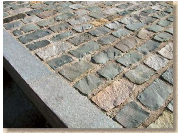
...can result in an uneven pavement
